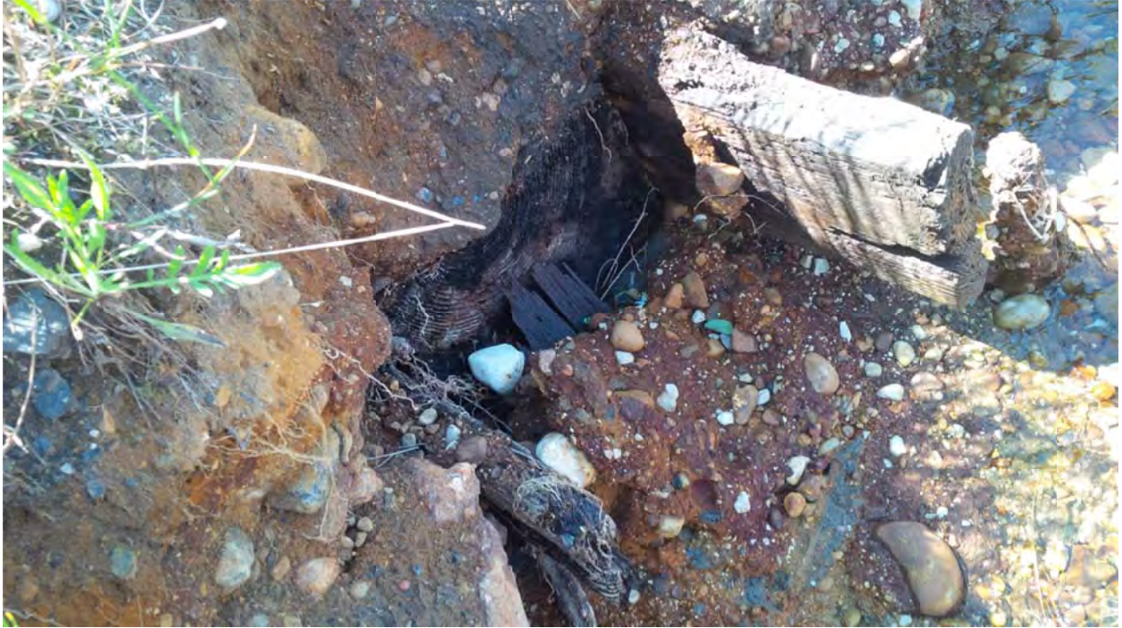
Photo 7: Remains of timber structure exposed in bank at east end of collapsed SSP wall section, East Reach
