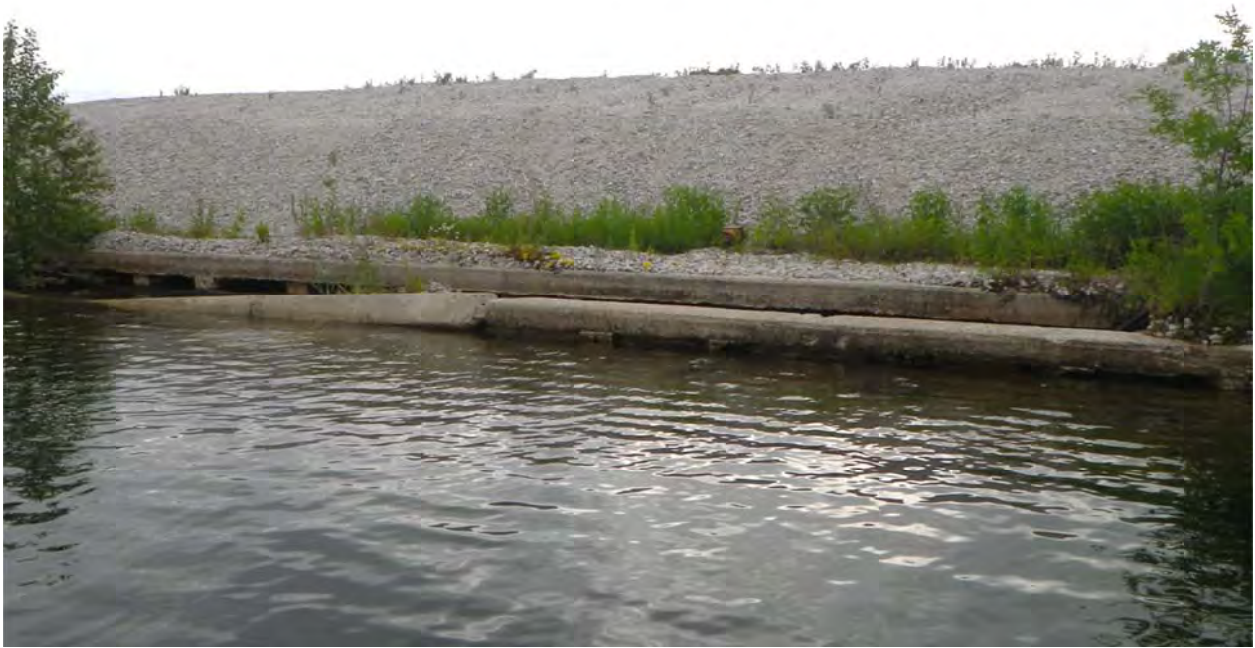
Photo 27: Exposed underside of concrete deck, west reach
