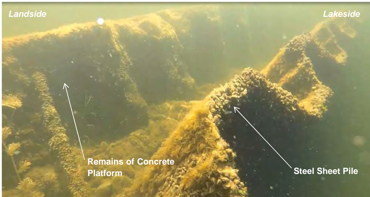
Photo 10: Collapsed SSP and Concrete Relieving Platform underwater (Day 1, Dive 1, 1:23:53)
