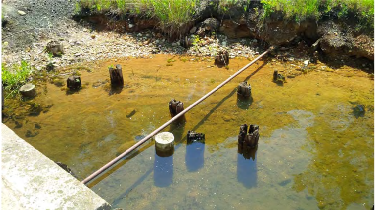
Photo 5: East end of collapsed SSP wall section, East Reach
