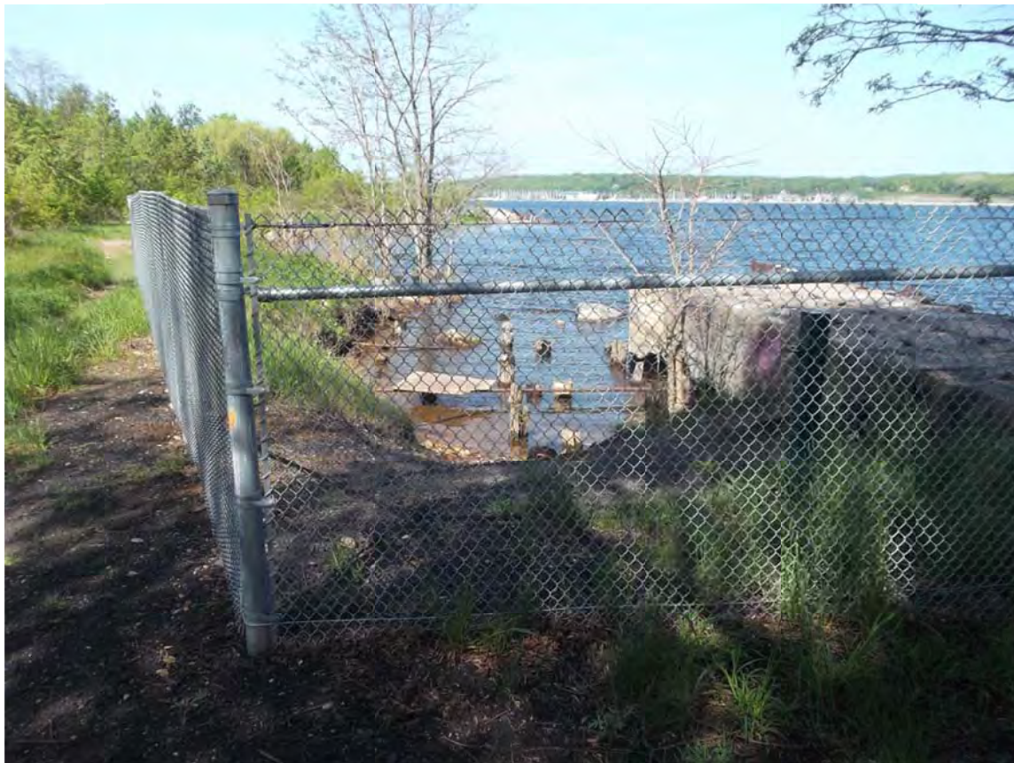
Photo 4: East end of collapsed SSP wall section, East Reach
