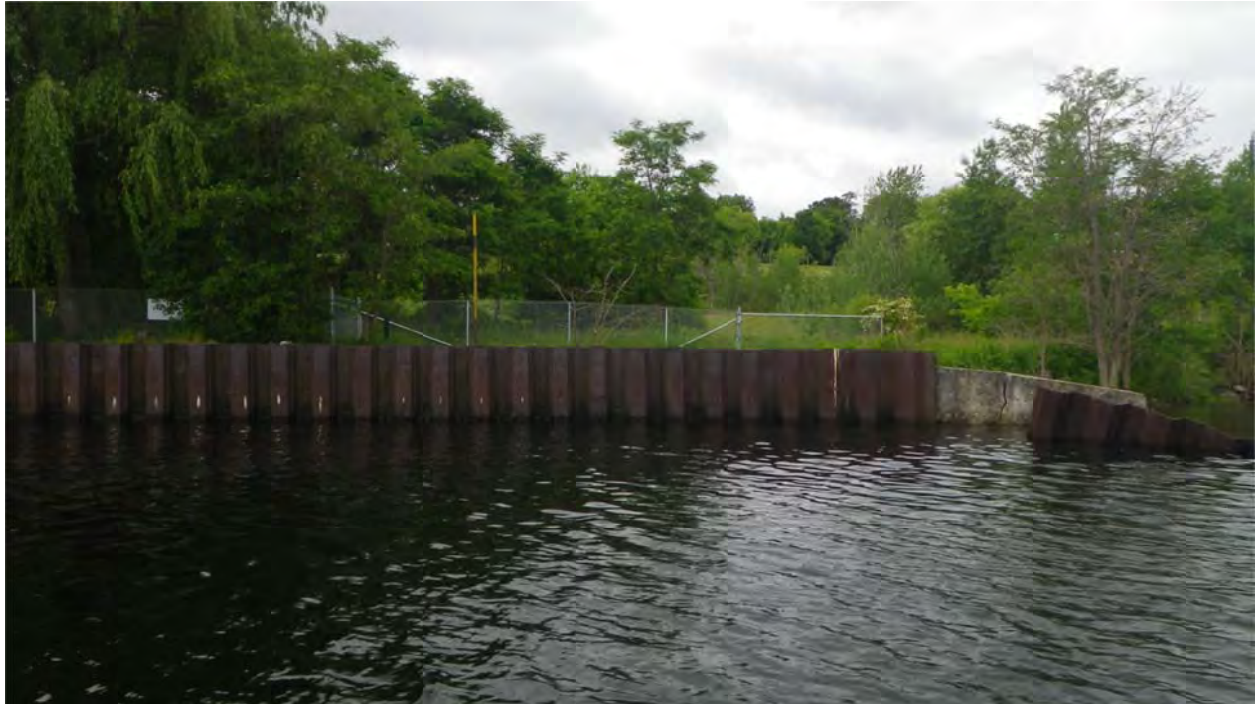
Photo 3: SSP wall at east end of collapsed section, East Reach
