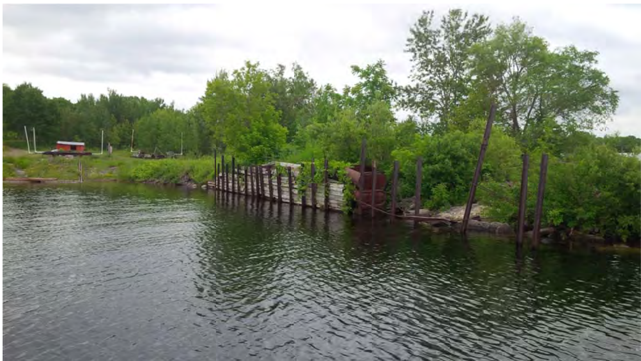
Photo 22: Remains of Pier, West side, Centre Reach
